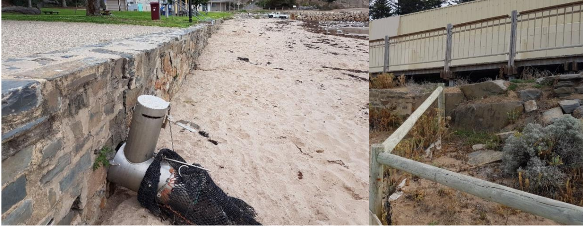
Figure 4: Stone wall fronting café cracking and rotated (left), Stone wall below board walk in poor condition (right). (Western et al., 2019g)
