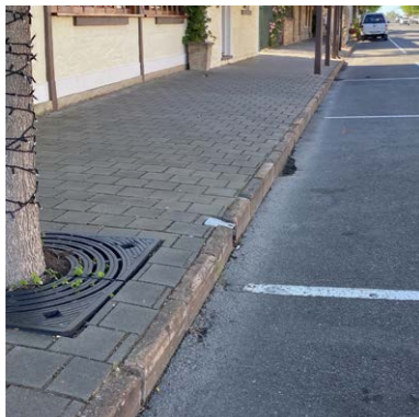
Existing red brick kerbing retained The historic red brick kerbing along High Street will be retained in all locations not affected by redesign of raised intersections
