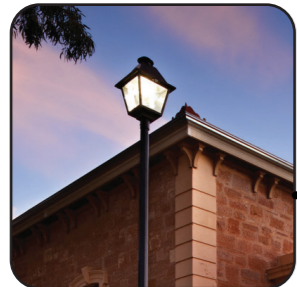
New street lighting with power supply for events
