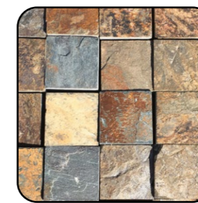
Cobblestone Banding in Road
