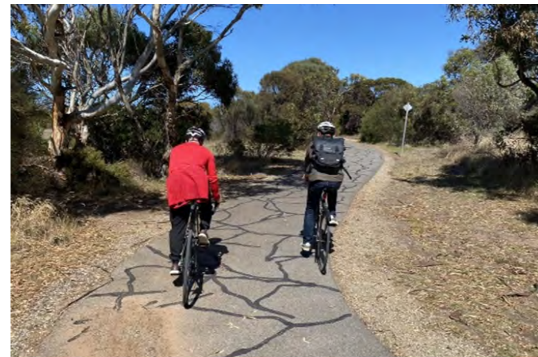
Deteriorated surface at Port Elliot
