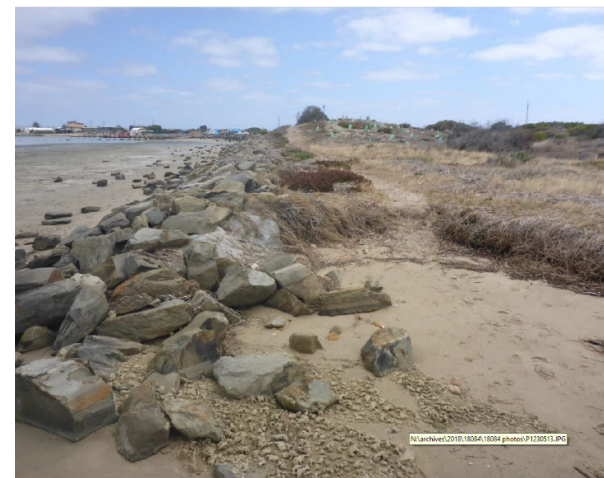
Figure 14- Erosion behind eastern end of the seawall.
