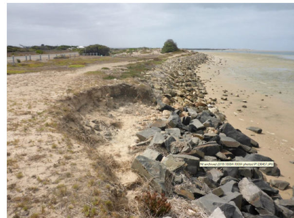
Figure 12- Erosion at the back of the existing seawall (eastern side of the boat ramp).
