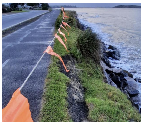
Coastal erosion at Yilki, Encounter Bay. Source: City of Victor Harbor
