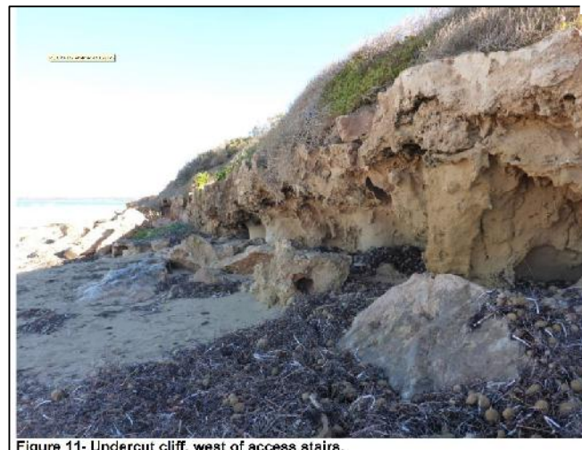
Figure 11- Undercut cliff, west of access stairs.
