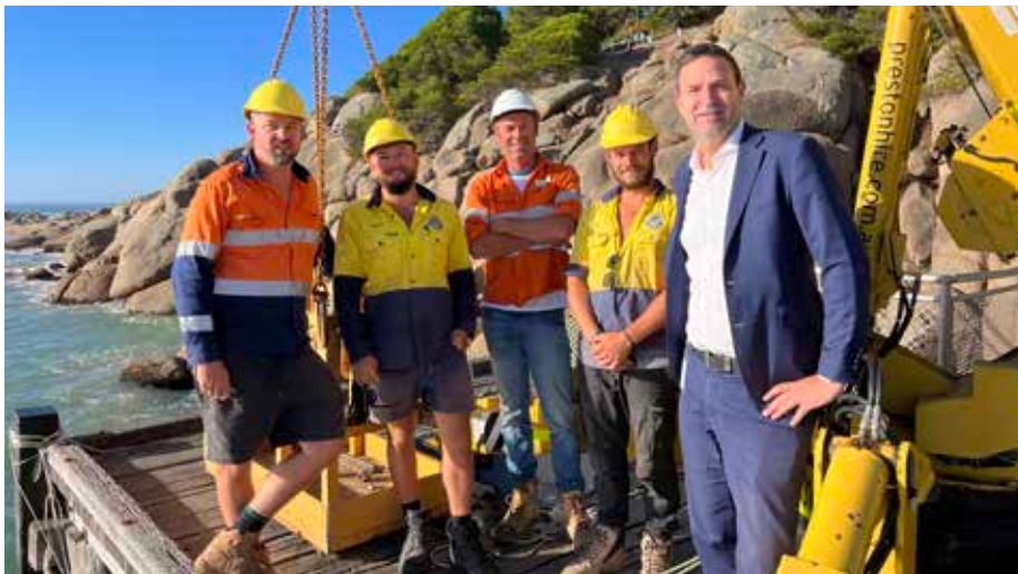
Image: Wiktor Boulden, Tom Thorne and Kadeem Welling from Queensland-based Aus Coast Diving have been installing new pylons with the help of crane driver Darren Ancell. They are pictured with Council CEO Nigel Morris (Courtesy of ABC - Caroline Horn)
